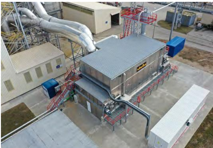
Broceni plant, Latvia: Type: BT 1/6200-13.5 – Product: RDF Dryer output capacity: 7.7 tph from 25 – 3% MC.
